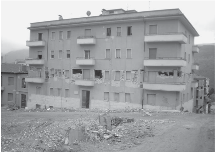
Plate 1. An example of incipient mid-floor failure in L'Aquila city
