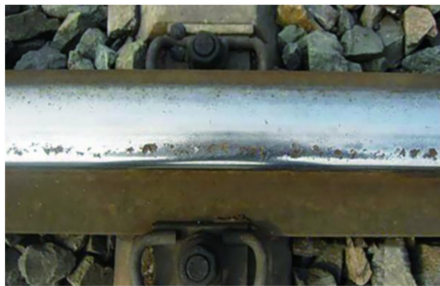
Curve section of the up track from Harbin West Railway Station of Wanggang-Sunjia Railway
