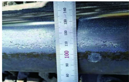
Curve section of the spiral-curve upper track at K496 of the border section of Harbin-Suifenhe Railway
